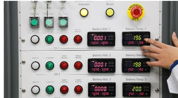
Voltage and Temp. Meter
